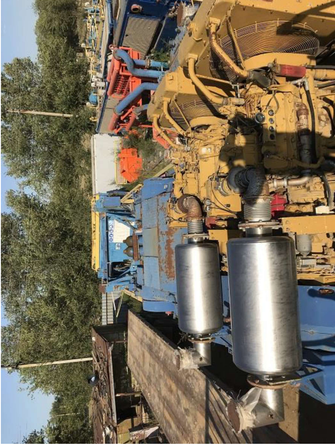
Photo no. 8 Caterpillar D398 Diesel Engine 2 pcs
